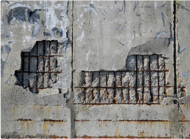
1. Active rebar corrosion
