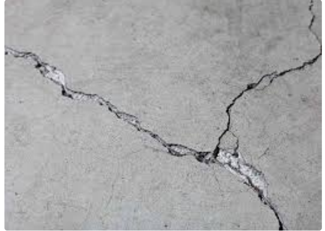
2. Surface-opening and internal cracks
